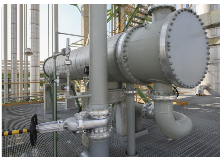
Scaled heat exchanger reduce functionality and increase cost.
