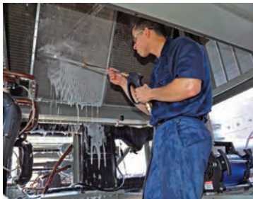
Clean thick coils inside and out
